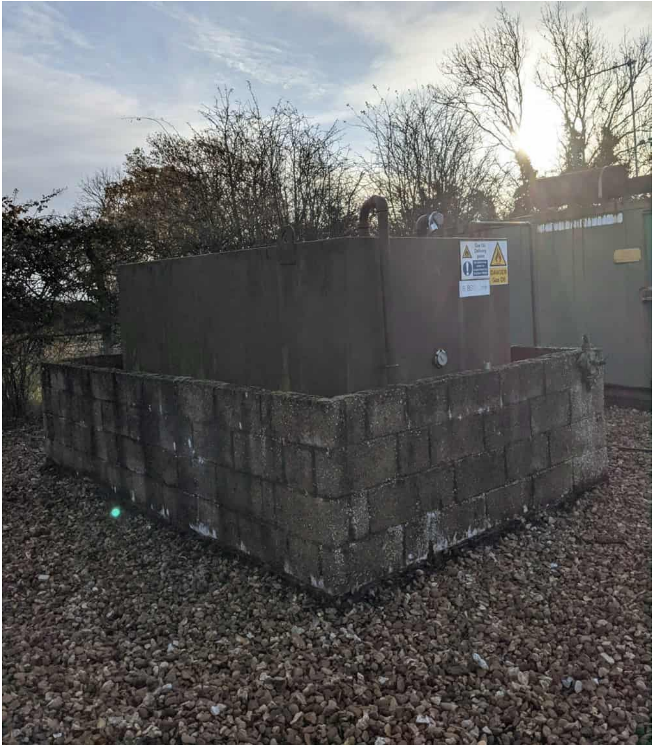
Photo 1: Waterbeach WRC fuel tank
